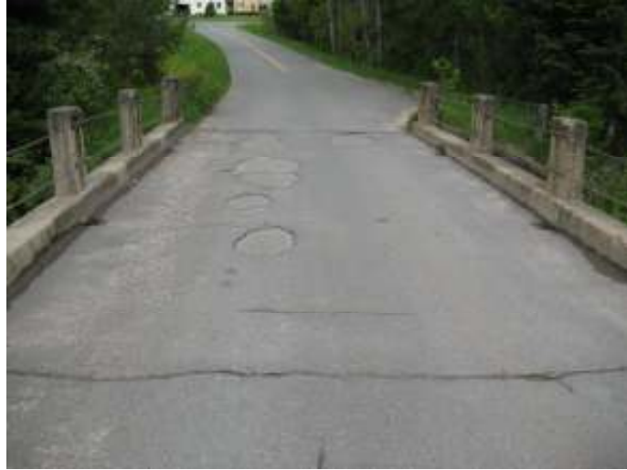
*pavement and membrane failure
