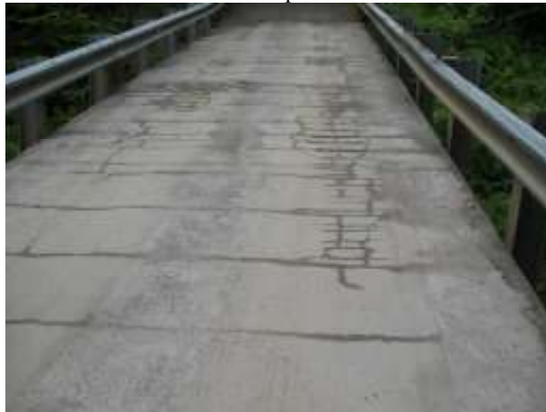
*deck cracking and leakage
