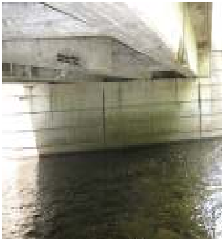
*concrete spall / visible reinforcement
