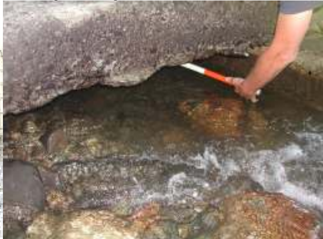
*undermining of foundation
