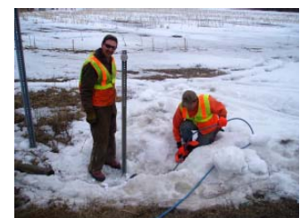
Thawing a frozen culvert
