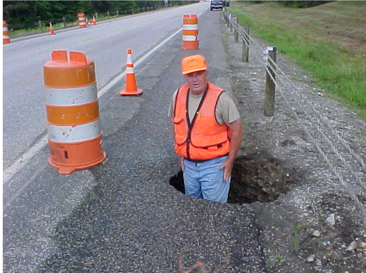
Culvert Failure in Sunderland on US7
