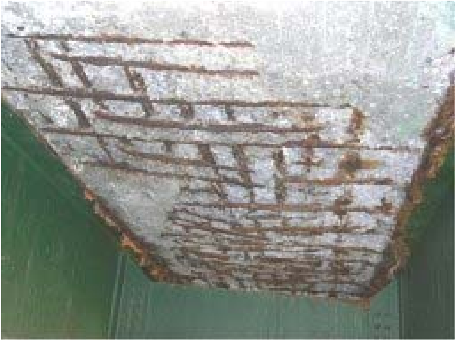
Underside of a concrete bridge deck – full depth holes on the horizon.
