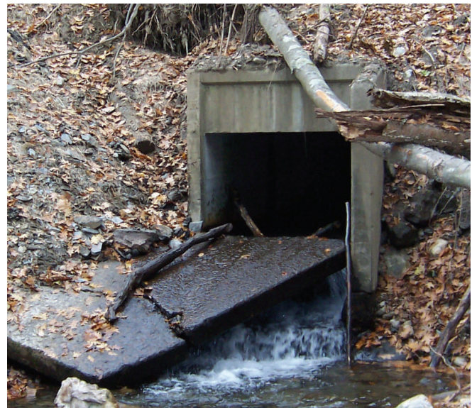
Small culvert rehabilitation has taken center stage in improving the condition of a critical asset
