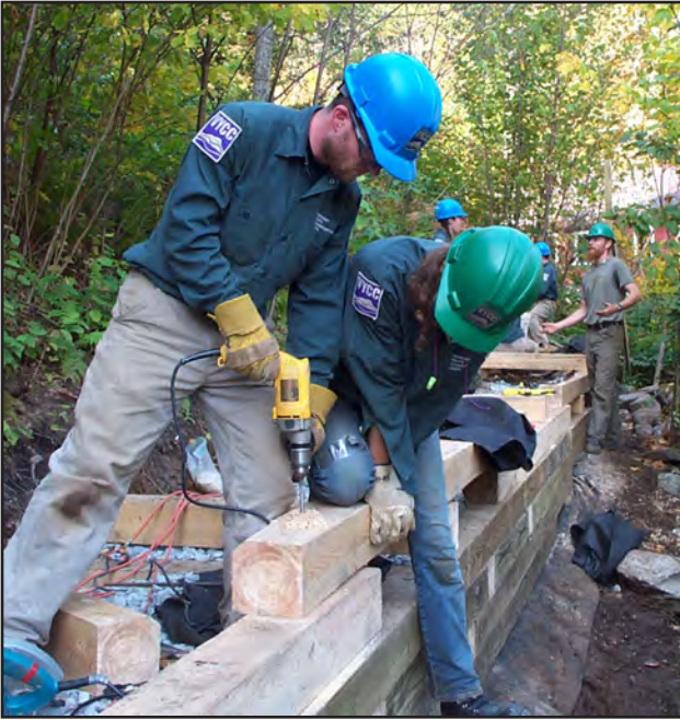
VYCC crews have constructed a 4-5 foot high elevated switchback trail that meets ADA standards for accessibility as part of the Thundering Falls reroute of the Appalachian Trail.
